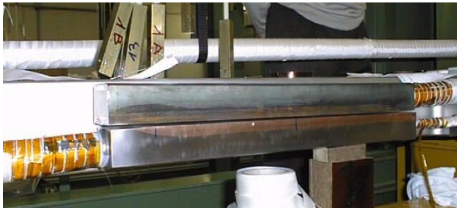
Fig. 5b: Two adjacent terminations of a DP module inner joint before being soldered and clamped together
